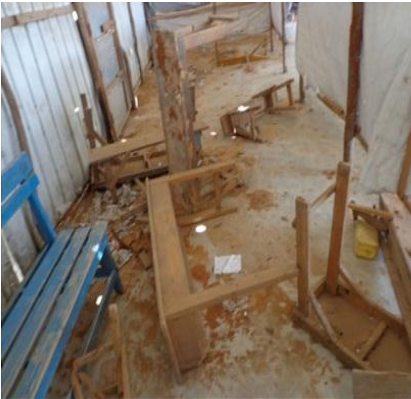
This school is half closed in Afgoye because of lacking rehabilitation
